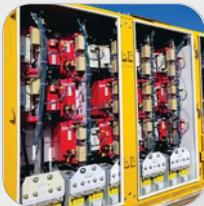
IGBT Control Panel
